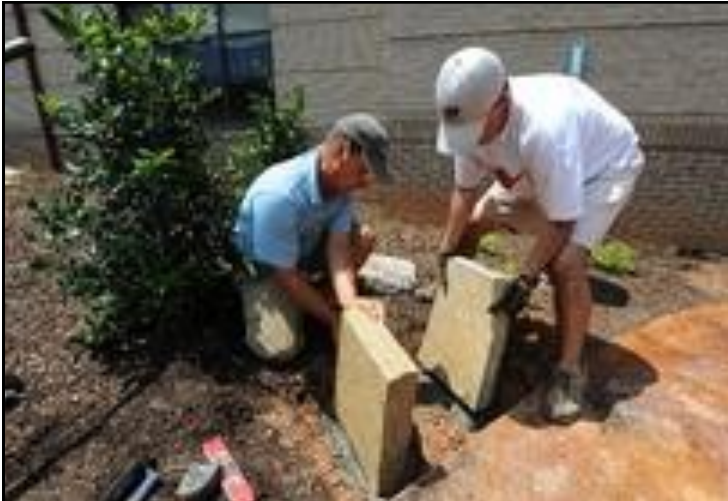
Johnny Crawford, Jcrawford@ajc.com States Wing and Jeff Bowling place stones in concrete as they build a stone bench inside the mini-farm classroom at Sharon Elementary School in Suwanee.
